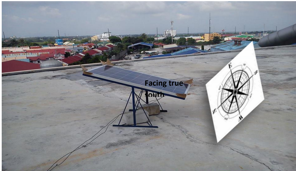
Figure 7: Location of the solar panel
